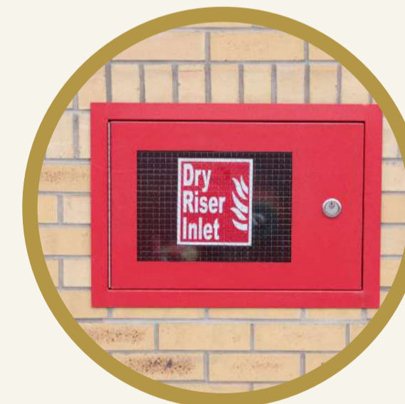
Equipment and access for fire services
