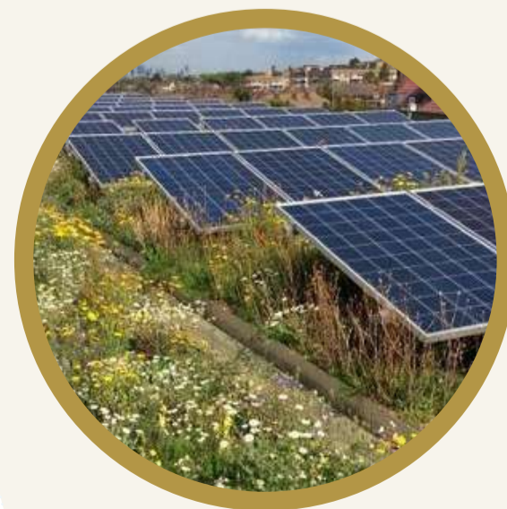
Solar panels on the roof
